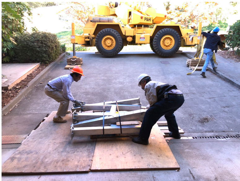
Vola works with members of facilities to transport the supports for the new ORNL equipment from the Chan Shun Loading Dock to the physics storage room.
